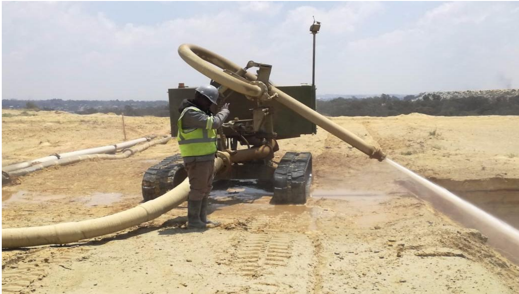
Figure 1: Mobile tracked hydraulic monitor on a tailings facility in South Africa
